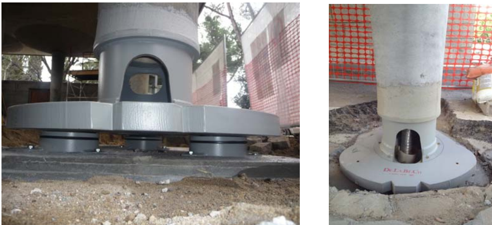
Figure 10. At left, support points at the base of tripods. At right, the internal flexible joint.
