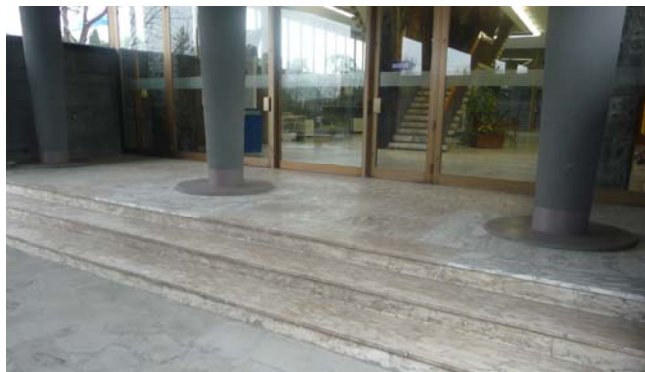
Figure 16. Final step of the work. The isolator devices are covered by metal protection cases.
