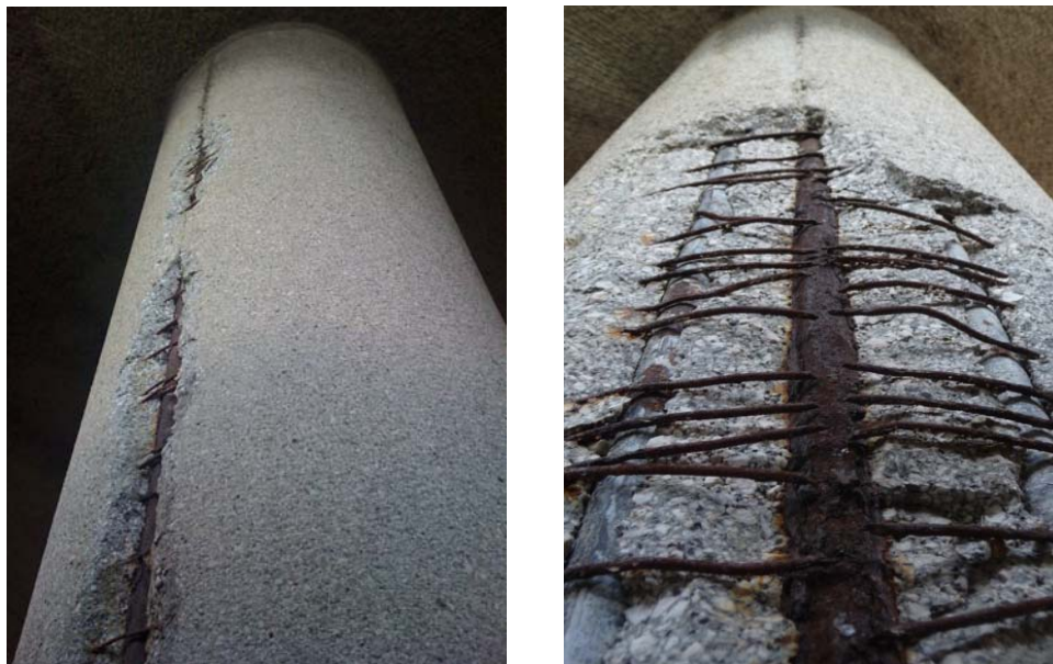
Figure 8. At left, mushroom shape column damaged by corrosion of bars. At right, particular of the high level of corrosion of longitudinal bars and stirrups.
