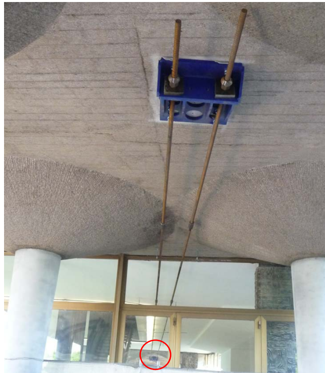
Figure 13. One of the two alignments of the displacement system control. With the red circle the anchorage of Est wing.
