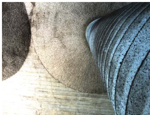
Figure 9. View from bottom of the column after the strengthening with CAM system.
