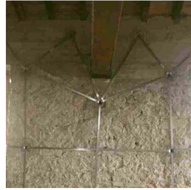
Fig. 12 - Detail of the link to the R/C kerb around a wooden truss.
