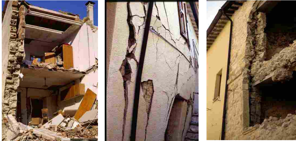
Fig. 1 - Collapse mechanisms of old Italian buildings (Umbria-Marche 1997 Earthquake).
