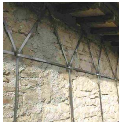
Fig. 9 – CAM arrangement in the facade and link to the top R/C kerb.
